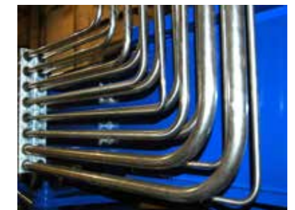
UV protected hoses & 316 stainless steel pipes and fittings
